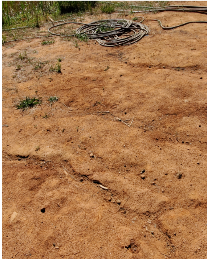
Figure 10. Erosion Example at Bummerville Reservoir
